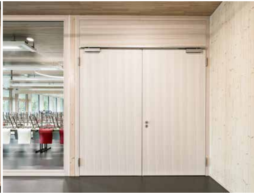
The double-leaf fire-rated door provides access to the cafeteria.
