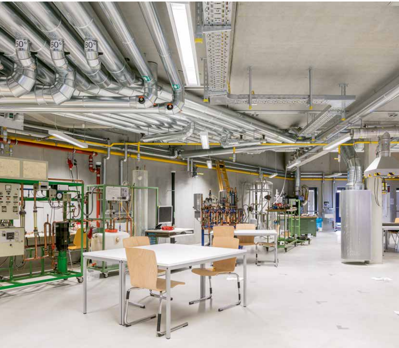
Lots of technology and space for experiments: The “seminar rooms” are geared towards practical test setups.
