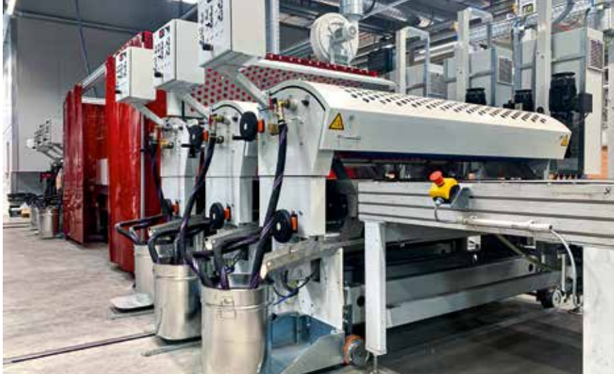
With the new coating system, Schörghuber can now switch between different coating techniques.
