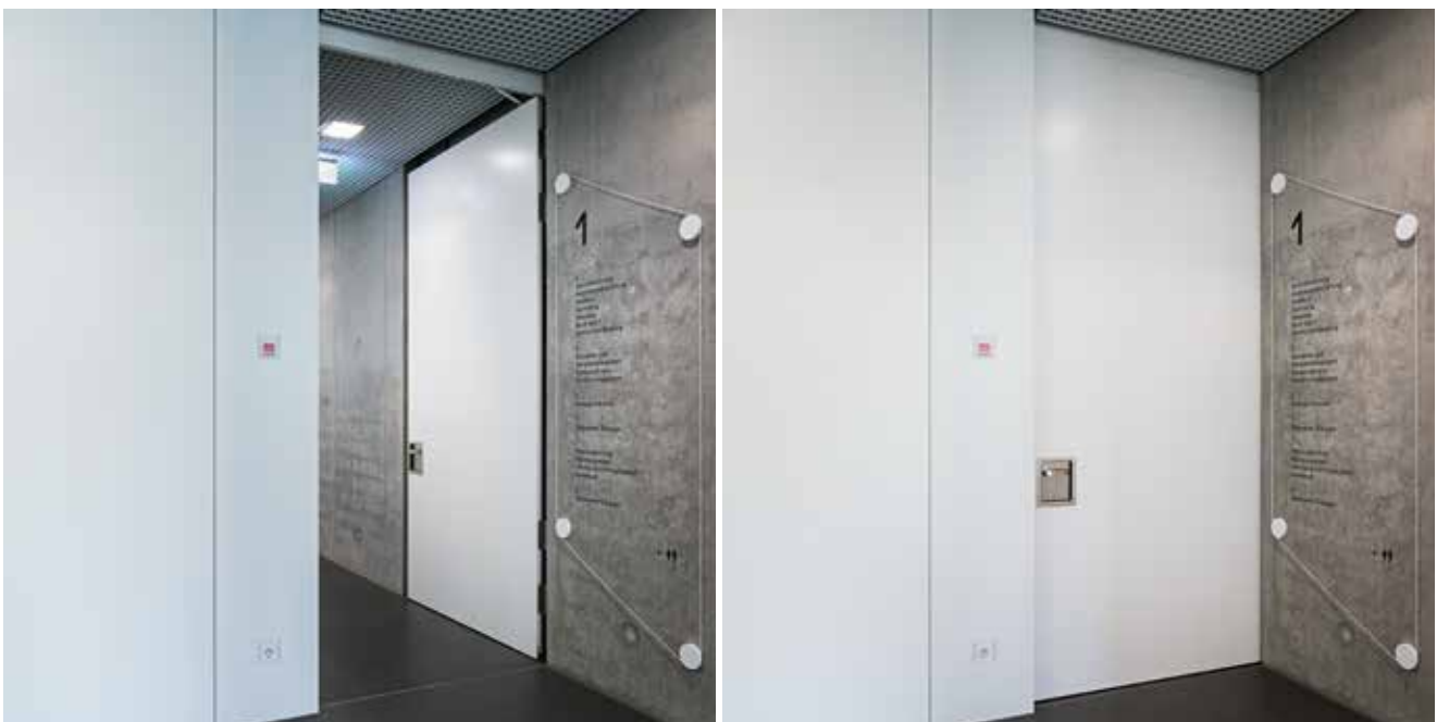
Recess doors “disappear” in the wall, offering a maximum passage width. These doors close automatically in case of a fire.
